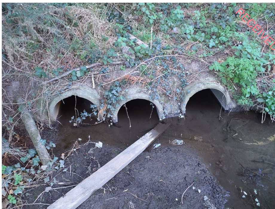
Plate 5-24: Culvert which the Corbally stream flows into directly north of the proposed development site.
